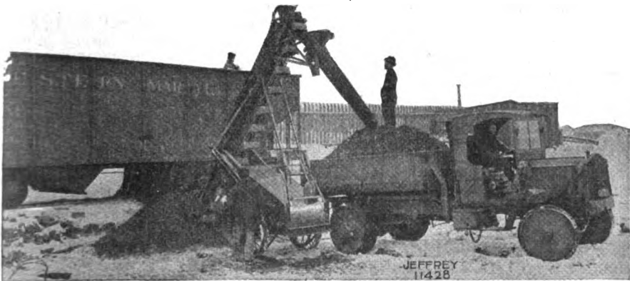
Loading direct from hopper bottom car into motor truck. Here a railroad tie has been removed and an extra man placed in the car to feed the material through the hopper doors.
